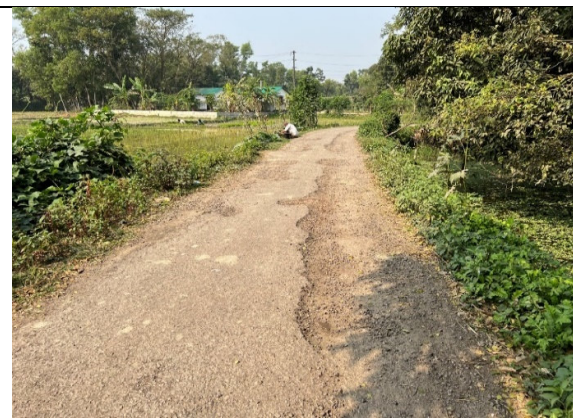
Road for rehabilitation: Chhatak Poursava
